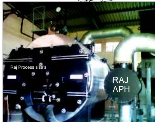
Husk Fired Boiler
